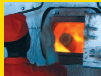
Wood specially grown to provide carbon-neutral energy fires the boiler at Unilever's tea estate in Kericho, Kenya. Unilever has been working with Kenya Forestry Research to increase the use of wood grown for fuel on the estate.
